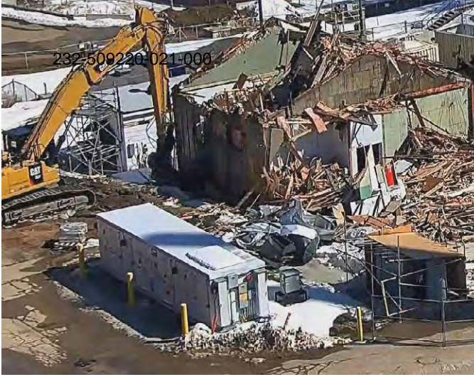
Building being demolished at the CRL site which will be disposed of in the proposed NSDF.
